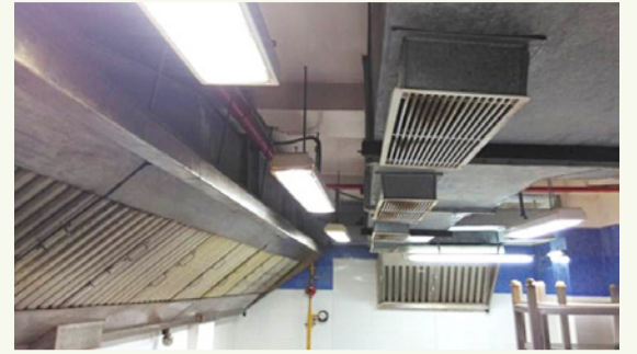
Kitchen air conditioning system
